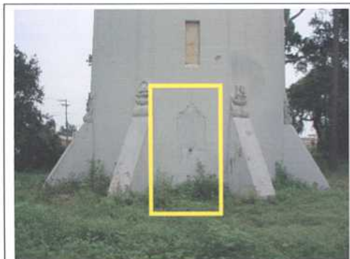
Figure 4.4 Several now-sealed doorways are seen between buttresses at the base of the tower.
